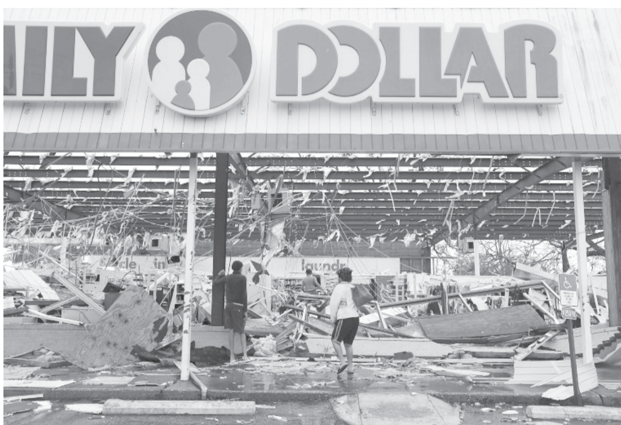
People look at a damaged store after Hurricane Michael ripped through Panama City, Florida. AFP
